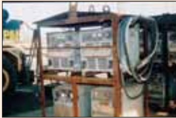
4 Pack Welding Station With (4) Lincoln Welders
